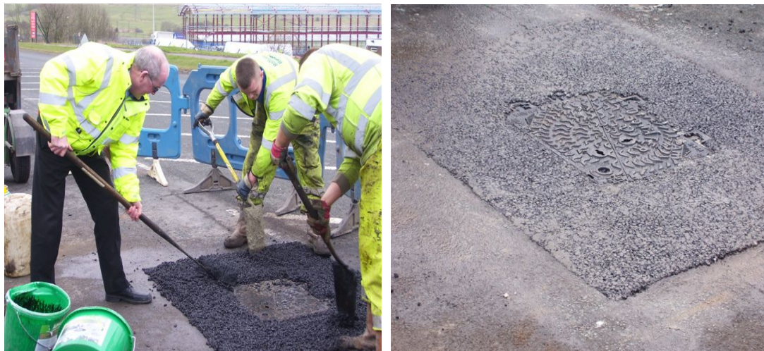
An example of Viafix being used for a utilities reinstatement on a class two dual carriageway
