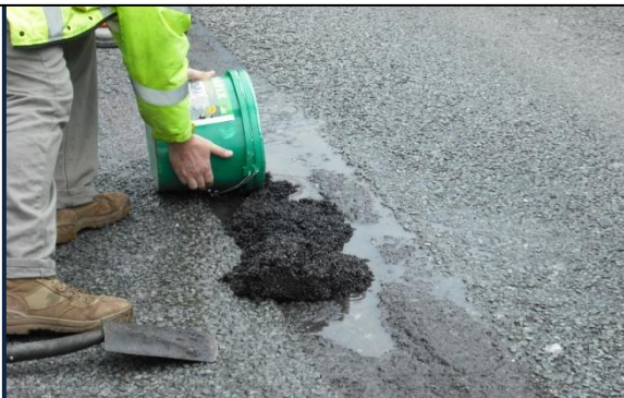
A permanent repair in freezing, wet conditions, without cutting or TM is possible with Viatec – Repair took 30 sec
