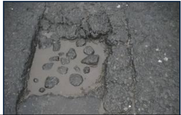
Dangerous pothole filled with standing water and debris – Viatec applied direct into water and broken asphalt
