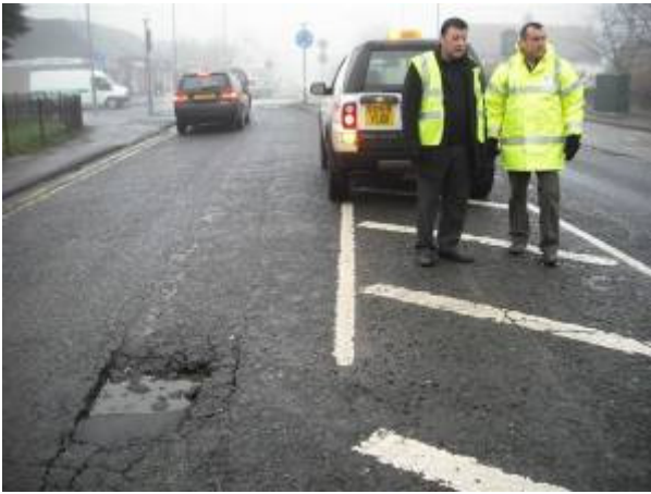
Catastrophic failure of trench reinstatement located in the wheel track (Nov 2009)
