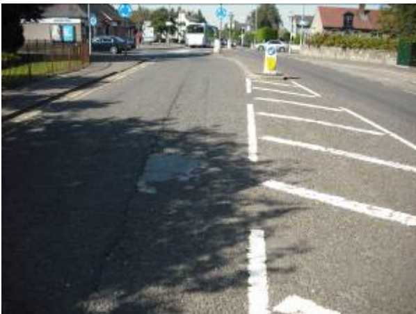
After Viafix was laid in foul weather, freezing conditions and trafficked immediately, it still stands in the road months later (Sep 2010)
