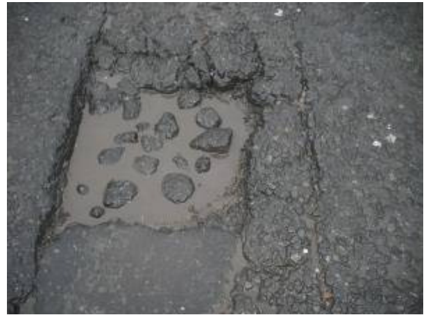
Dangerous pothole filled with standing water and debris – Viafix applied direct into water and broken asphalt
