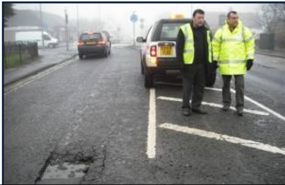
Catastrophic failure of trench reinstatement located in the wheel track (Nov 2009)
